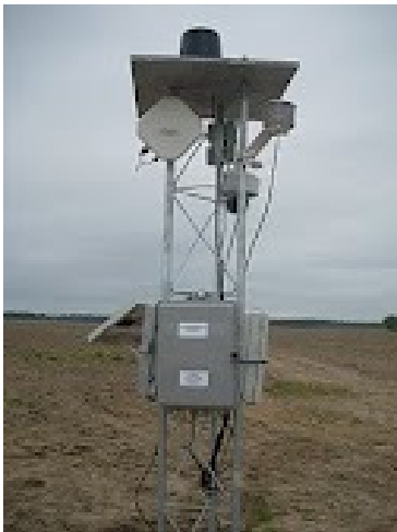
Wireless Solar Base Station
